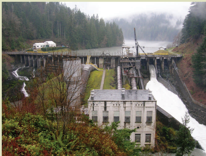
It is expected that the dam removal will be finished in March, 2014.
